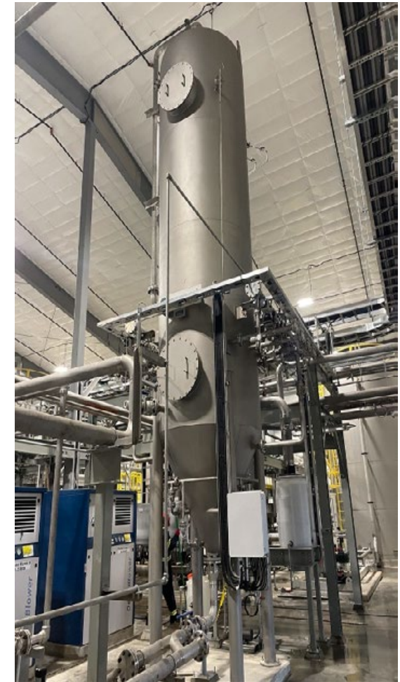
Sulfur Mitigation System
